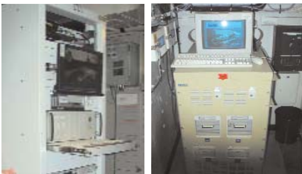
Figs. 7 & 7A: Original and latest in server cabinet design – the latter allows for more capable contents
